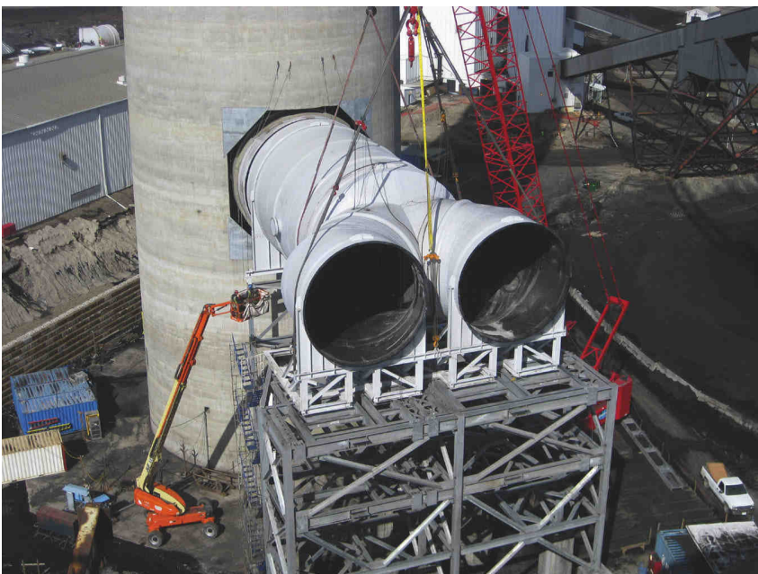
That's no Space Shuttle exhaust, that's large spool FRP ductwork made with Ashland's HETRON epoxy vinyl ester resin and glass for a North Dakota FGD system. Ershigs filament wound the 21-30 ft diameter components.
