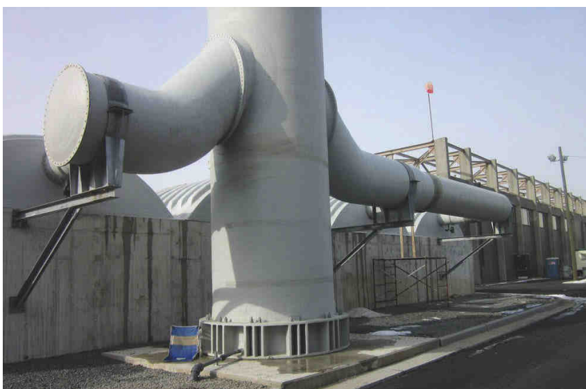
For a New Jersey odour control system, FRP ductwork built by ECS using AOC Vipel vinyl ester resin and Owens Corning glass helps move 3400 m 3 per minute of air and saved the end user 60% in component costs compared to stainless steel equipment.
