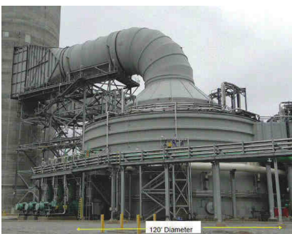
Success story for FRP: Ashland's glass-reinforced resins offer corrosion protection in the scrubber and ductwork equipment that is part of one of the largest jet bubbling reactors in North America, installed at a 950 MW power plant.
