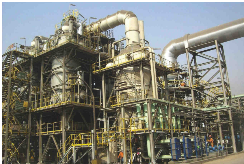
Minerals processing is a growth area for FRP. At the sulphuric acid plant that is part of Votorantim Metals' zinc refinery in Cajamarquilla, Peru, FRP scrubbers, tanks, piping and ductwork are made using Ashland's Derakane epoxy vinyl ester resins.
